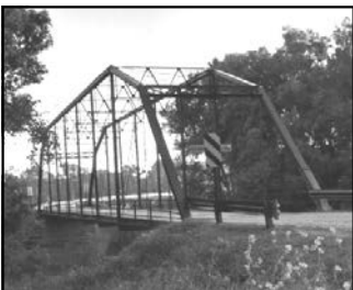
Dodd Ford Bridge (Bridge No. 1461), County Highway 147 over the Blue Earth River, Shelby Township (vicinity of Amboy)
