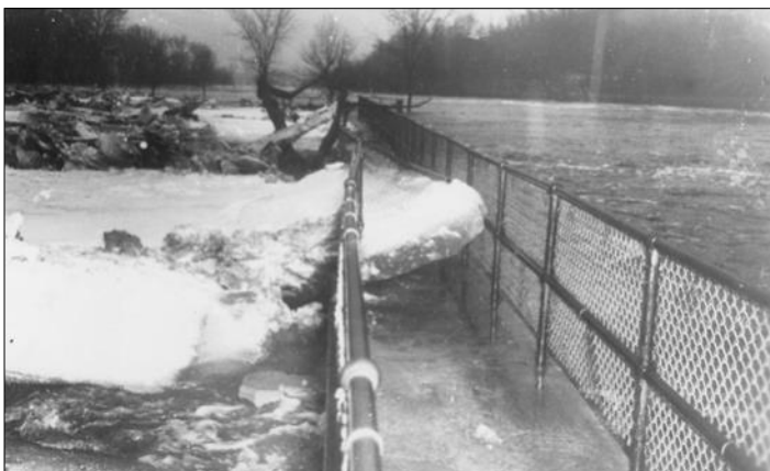
Ice chunks pushed through the fence on the dam's walkway during the 1951 flood
